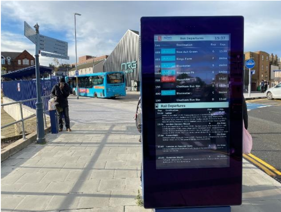
Figure 32 Digital signage screen outside Gravesend Station showing real time rail and bus information. Source: Network Rail
